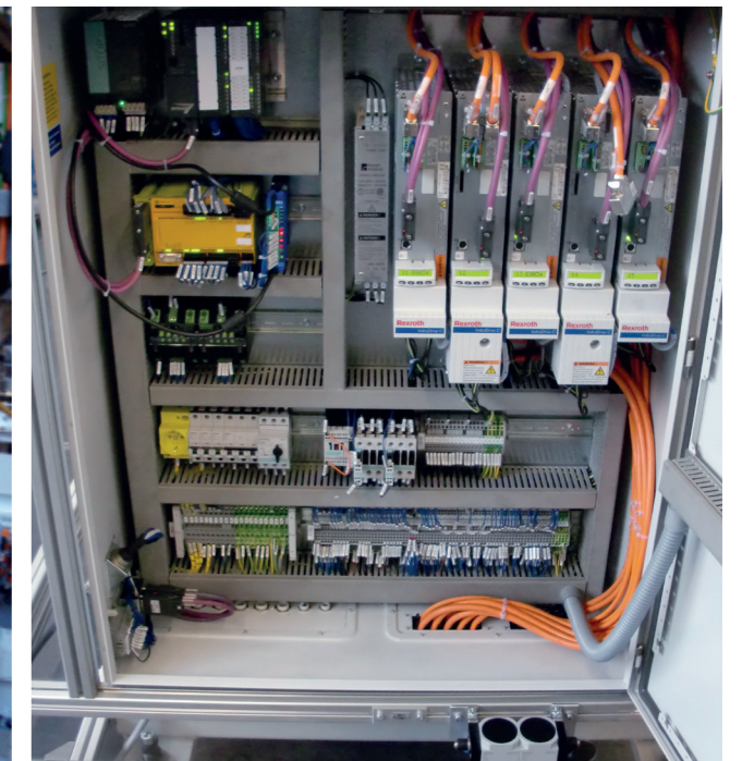
>> Switch cabinet view
